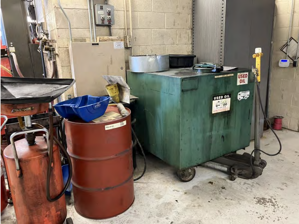
Photo 13: Drums and used oil AST in the east garage bay
