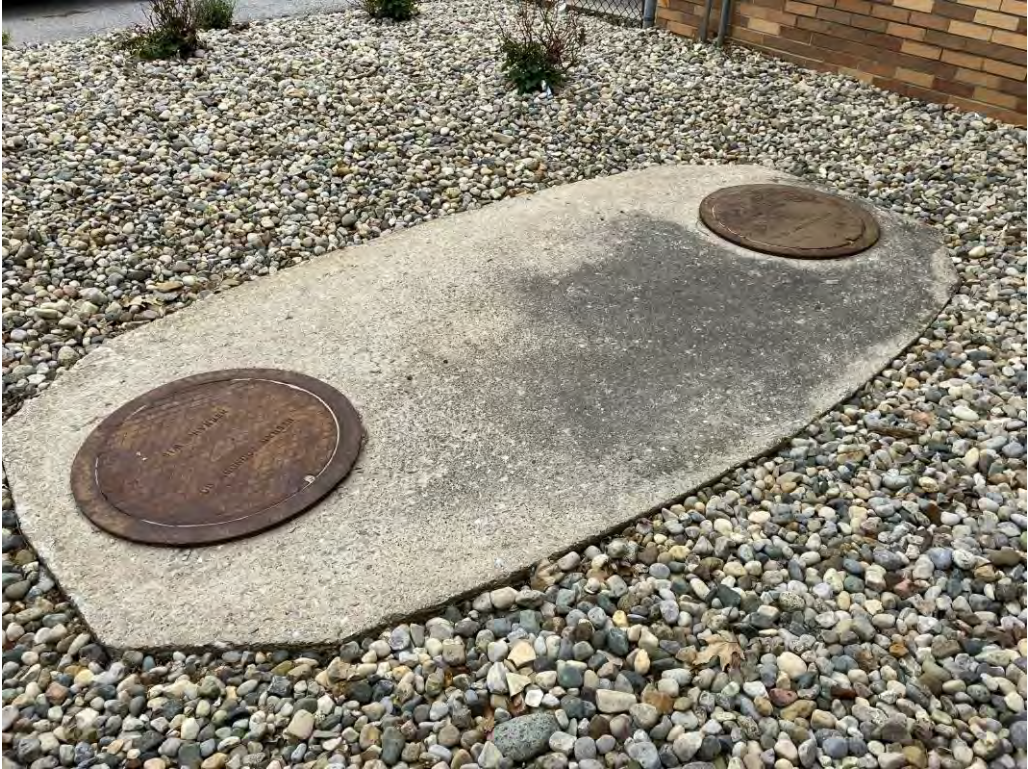
Photo 15: Oil/water separator south of the building
