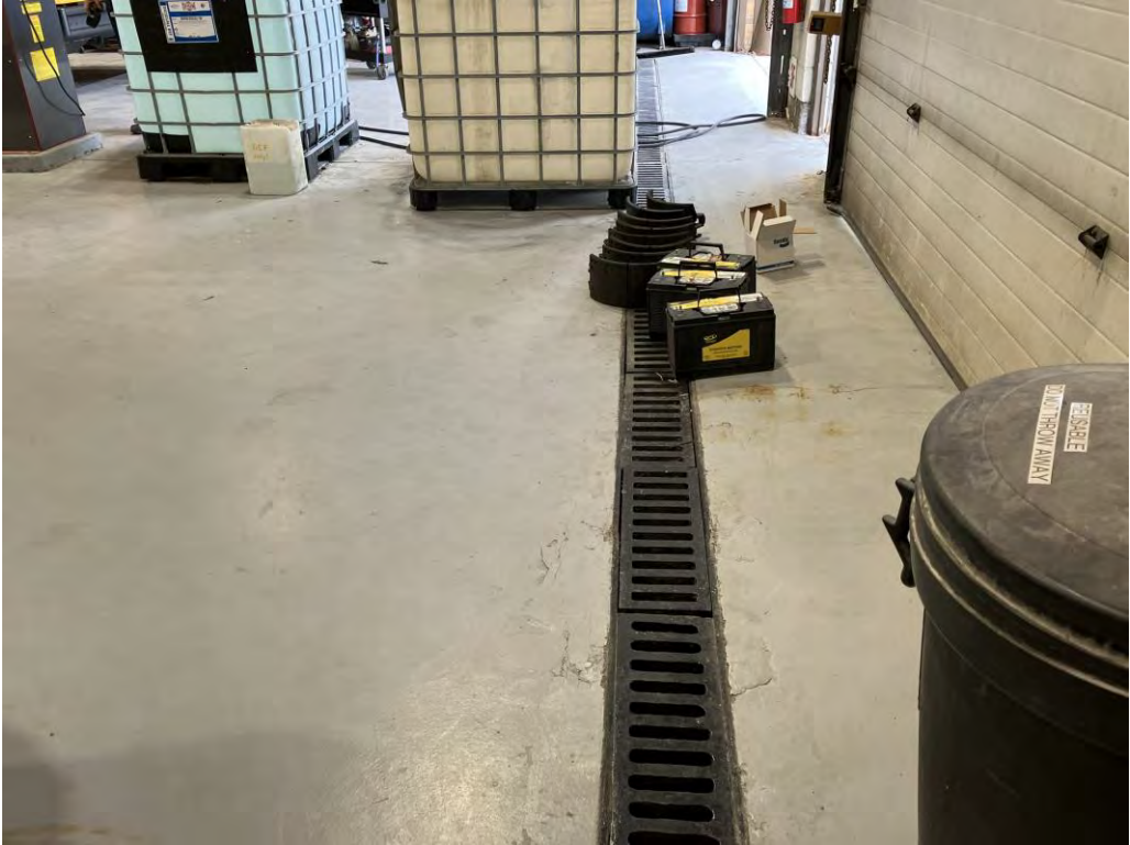
Photo 17: Trench drain at the service bay
