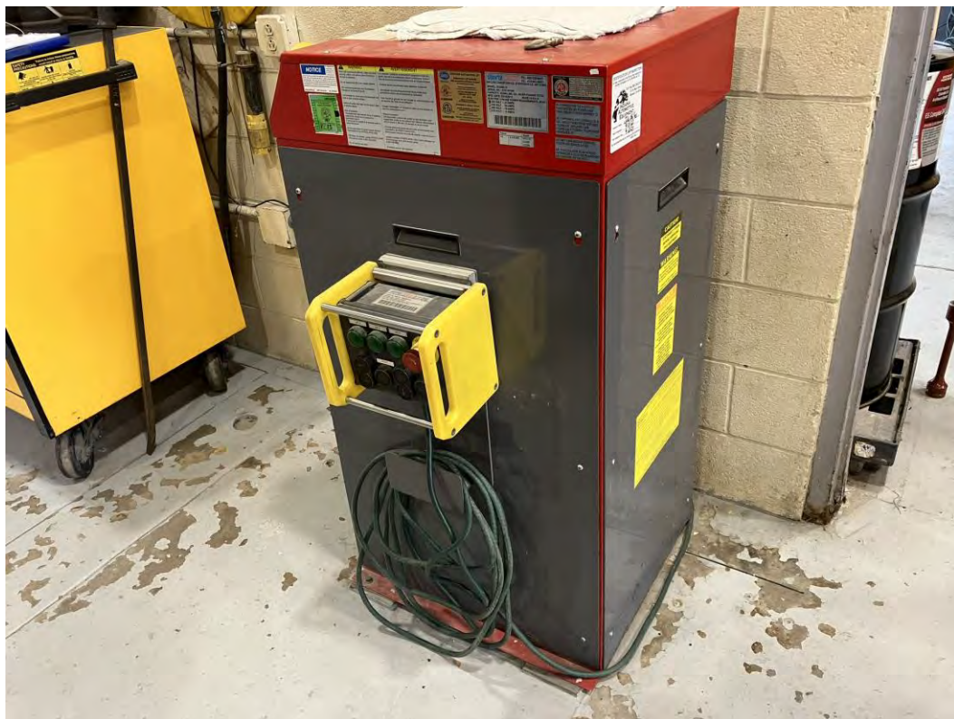
Photo 22: Hydraulic reservoir and controls adjacent to pit lift
