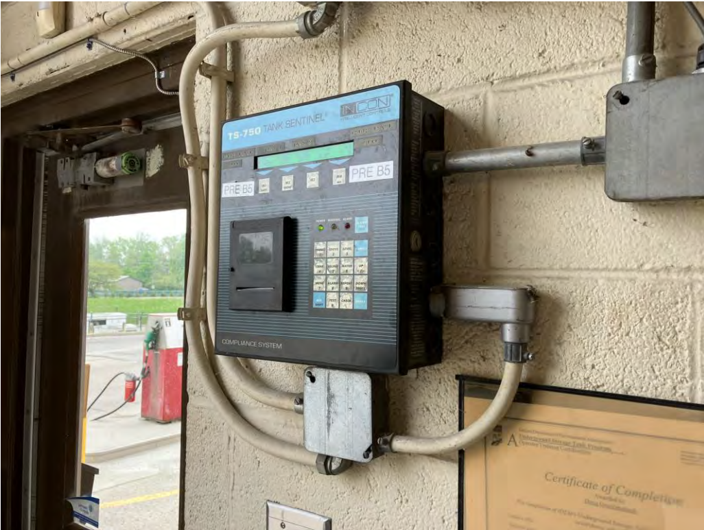
Photo 38: UST ATG in the office
