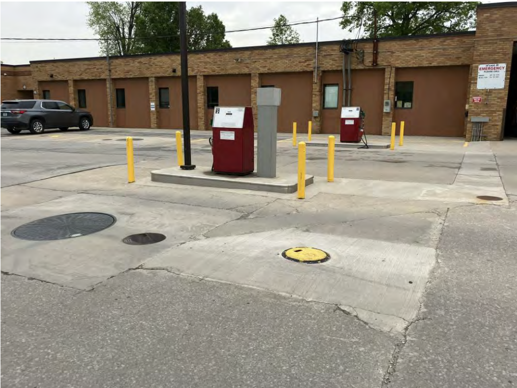
Photo 32: UST area and fuel dispensers north of the office/garage building
