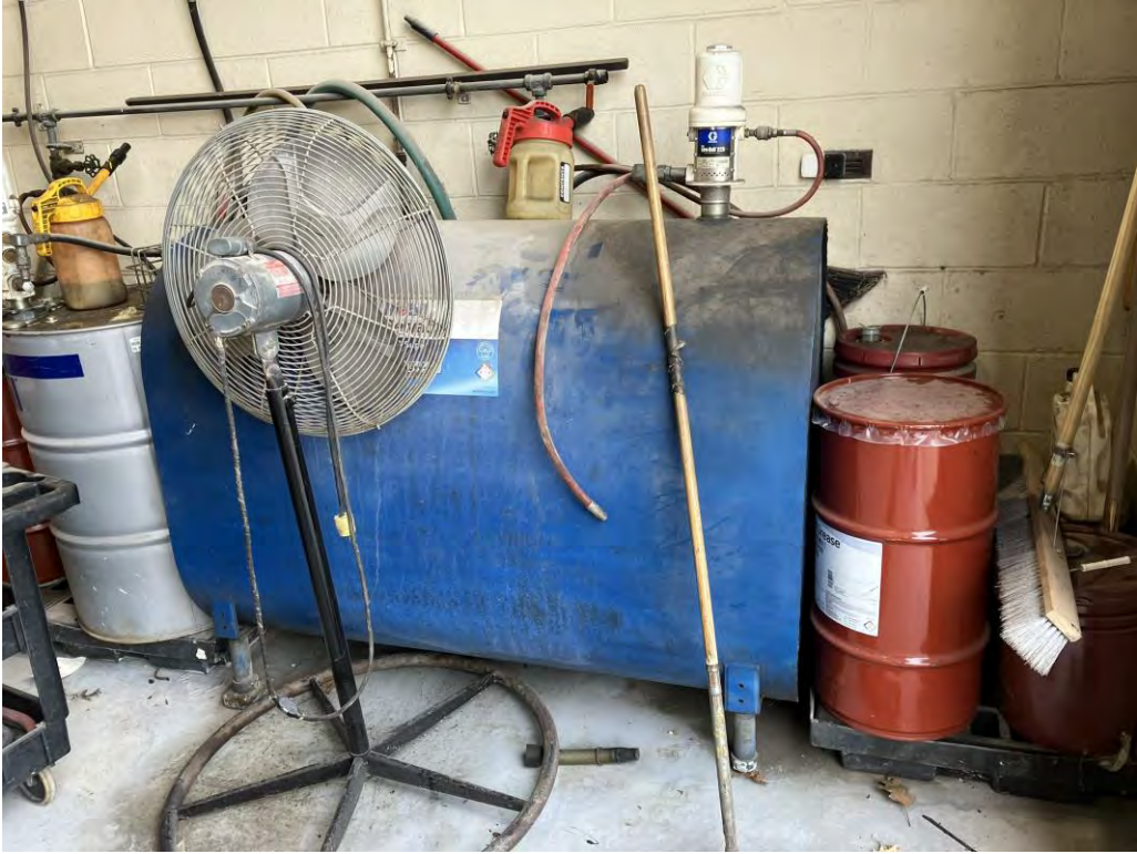
Photo 19: Oil AST, grease drums, and oil drums at the service area
