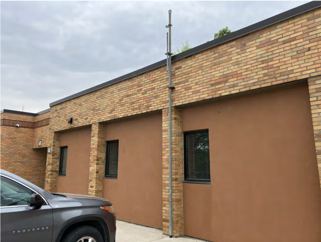
Photo 34: UST vent pipe
