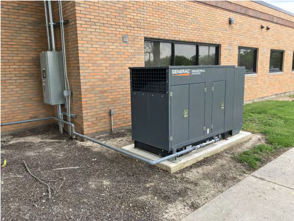
Photo 39: Emergency generator located south of the building
